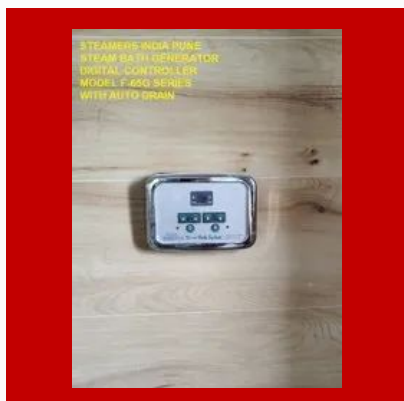
Steam Bath Sauna Bath Jacuzzi And Chill Shower Installations
